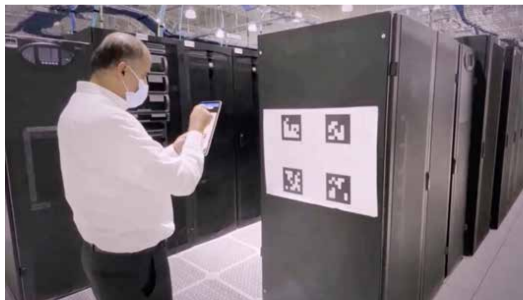
By scanning QR codes in the IT Corporate Data Center, a new augmented reality tool allows users to locate, verify, and discover key information about assets in the IT Corporate Data Center.
